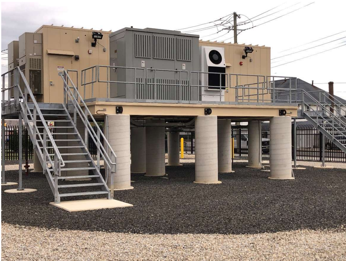
Figure 2. Exterior View of the Beach Haven BESS. Reproduced from [1].
